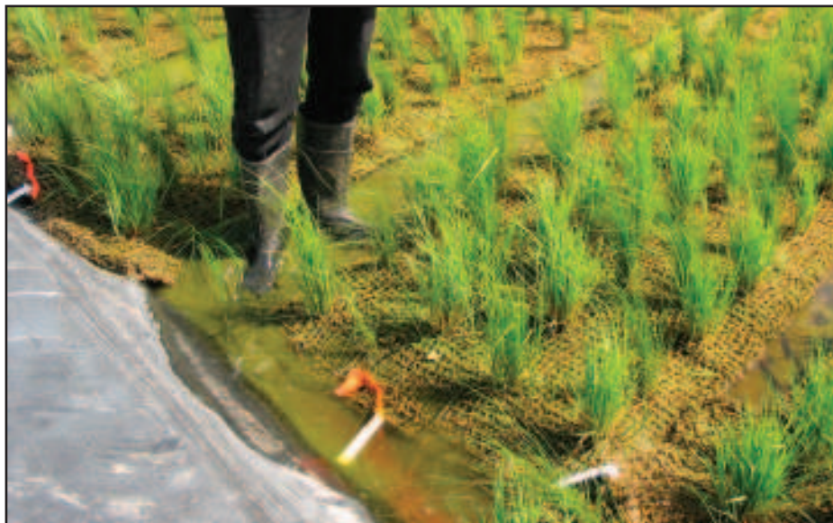
The pre-planted erosion control mat is grown with native plants to produce maximum root growth.
