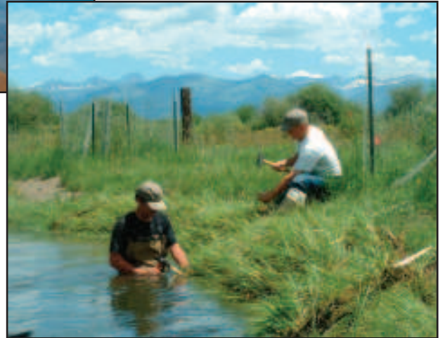
Top: Construction of the first soil terrace. Lower: Site conditions during Wetland Sod installation.
